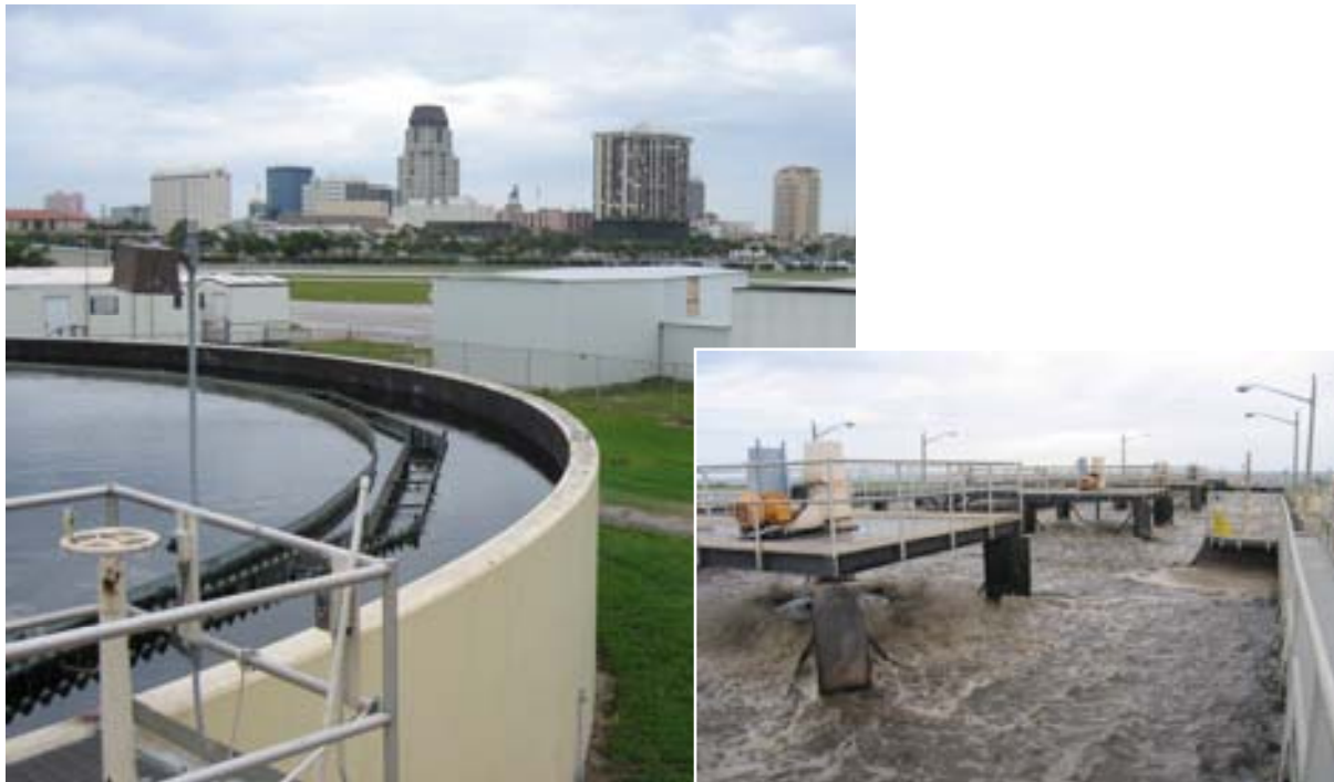
Figure 17 Aerators and clarifiers at St Petersburg WRF, showing St Petersburg in the background.
