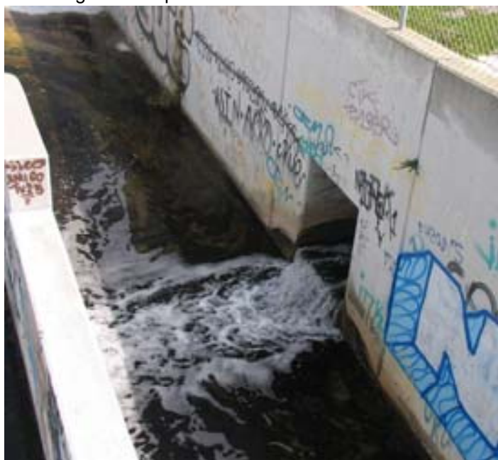
Figure 28 Discharge from water treatment facility's R/O plant entering a stormwater drain, Sweetwater, San Diego.
