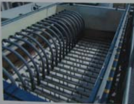
The submersible microfiltration membranes operate continuously, removing particles and bacteria and improving the overall water quality.
