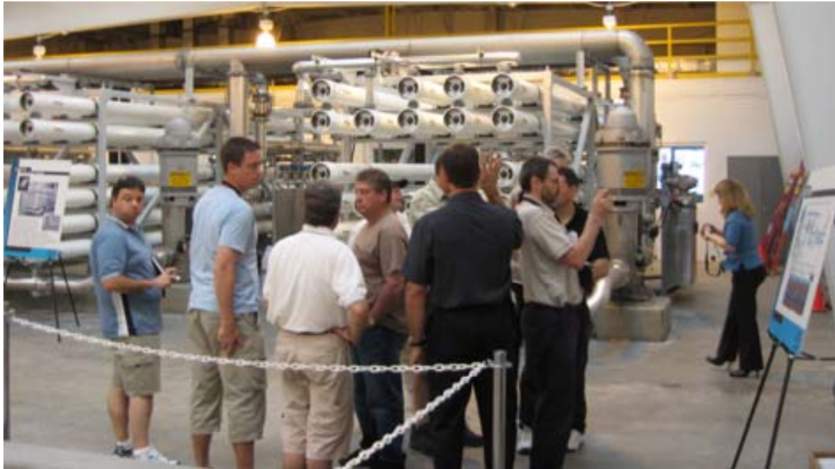
Figure 29 Desalination plant, Sweetwater, San Diego, California.
