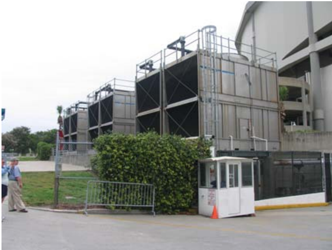
Figure 19 St Petersburg Sports Dome cooling towers.
