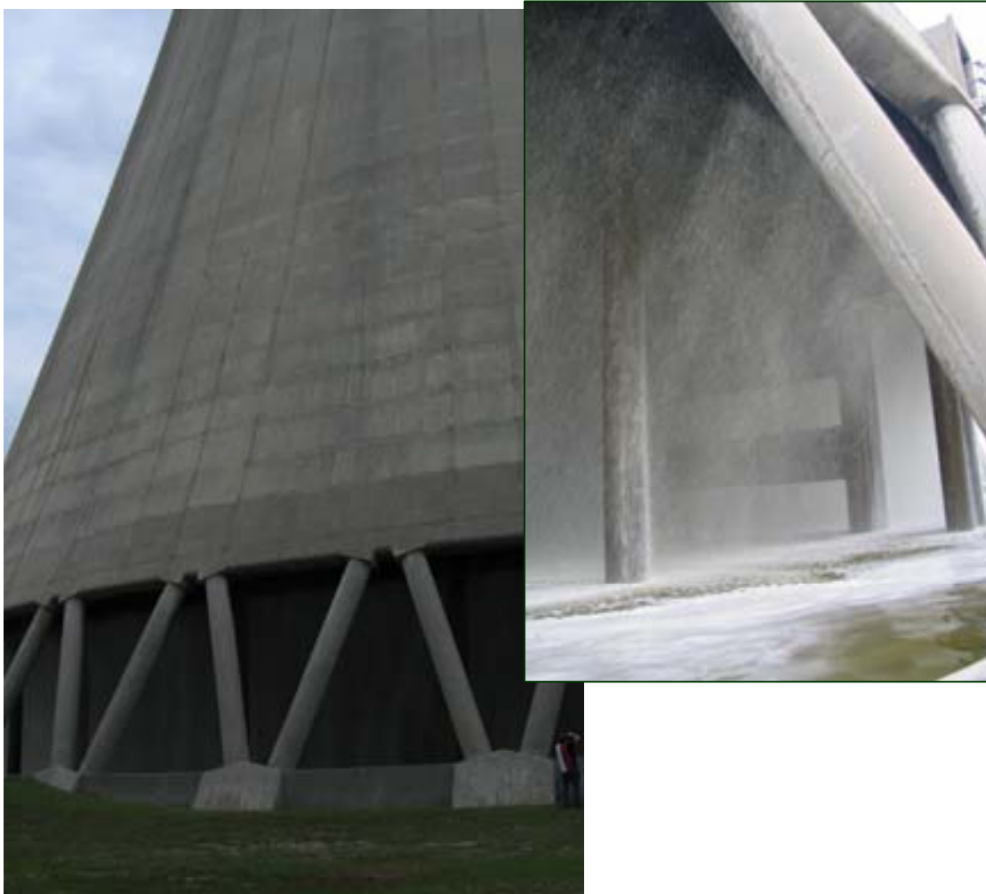
Figure 5 Recycled water used in a cooling tower at the Orange County Power Station, Florida.
