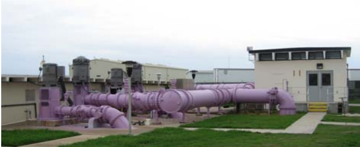
Figure 16 Recycled water pumps at the St Petersburg WRF, Florida.
