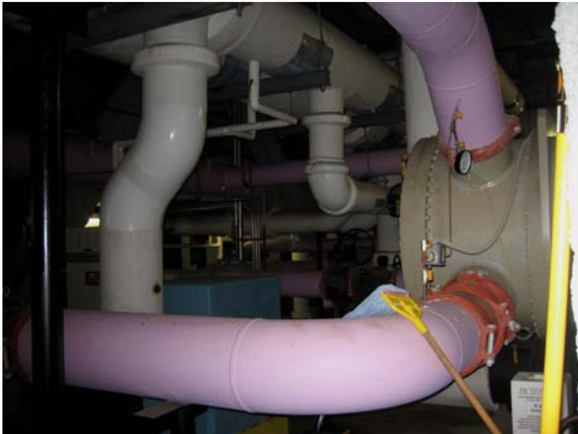
Figure 18 Chiller units and piping linked to cooling towers at the St Petersburg Sports Dome.
